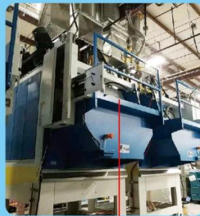
Service platform This structure provides a safe work environment for operators.
